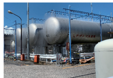
Water cooling system for LPG tanks
